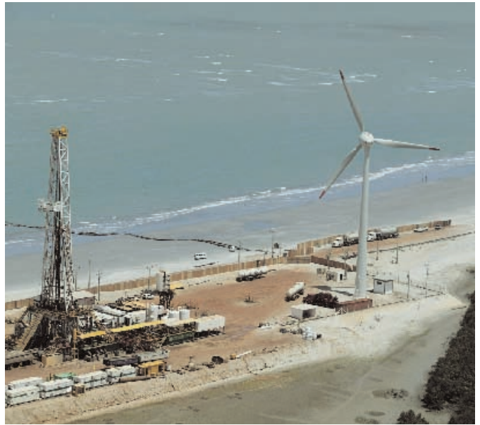
A wind turbine tower is being installed in Macau in the State of Rio Grande do Norte. Petrobras recently inaugurated its first pilot wind project with an installed capacity of 1.8 MW (Petrobras)
