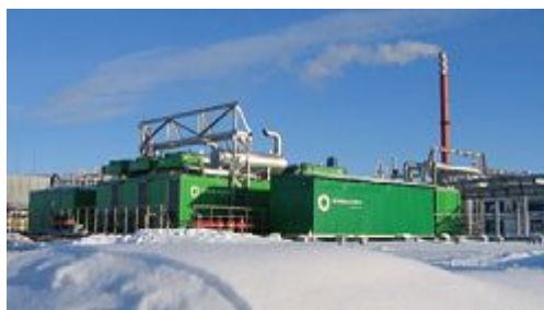
Three Jenbacher natural gas-fired units operate in island mode in Yamal-Nenets Autonomous Region, a major gas producer in Russia's far north (GE Jenbacher)
